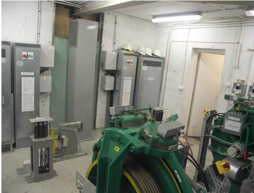
Fig. 3. Machine room with installed gearless winches MX18 with the friction pulleys 690 mm in diameter [3]
